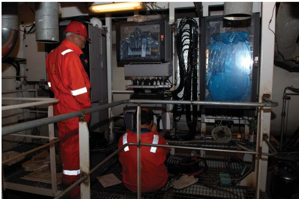
Photo 9. The transceiver and preamplifier units for EM120 and SBP120. These were installed above the engine room on a specially constructed platform.
